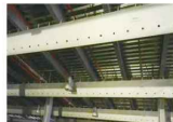
宁波新源科技车间通风项目 Ningbo New Energy Science and Technology Workshop
