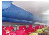
聚丰祥食品保鲜车间降温项目 Cooling Project of Jufengxiang Food Pickle Workshop
